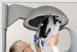
6. Remove the gear tray and replace with a new LED generation gear tray
